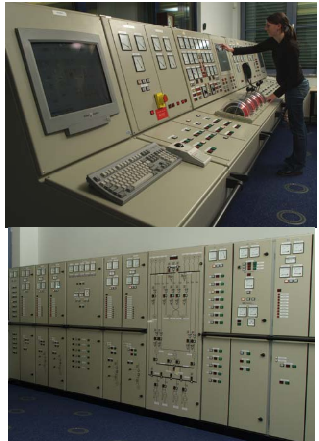
Fig. 8: SES Control room: Electric switchboard of Full Mission Ship Engine Simulator with Medium Voltage panel in the centre (bottom) and engine operation panel (top).
